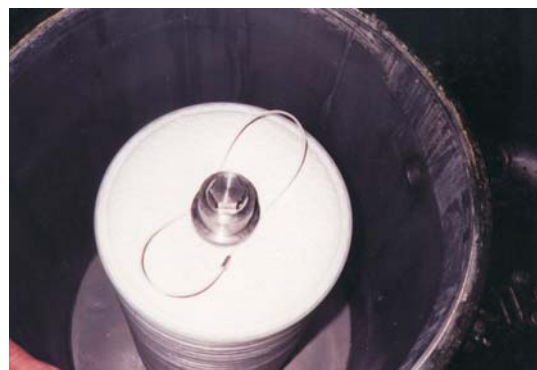
Figure 7. - Zeta Plus Cartridge Installed
